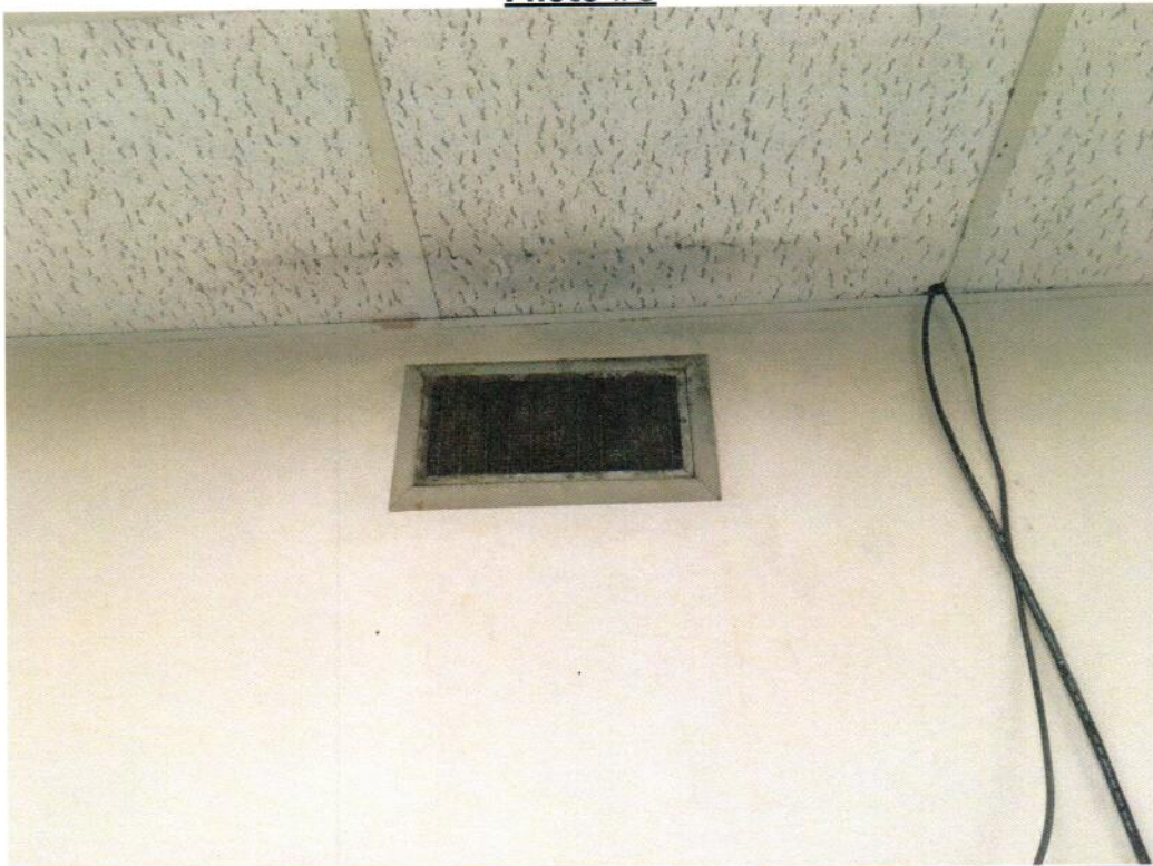
State of Hawaii DOT Highways Penthouse Supply register with particulate accumulation.
