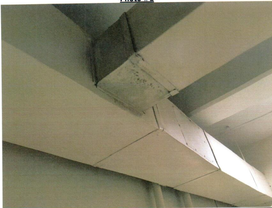
State of Hawaii DOT Highways Penthouse Mold accumulation due to condensation on ductwork outside of penthouse entrance.
